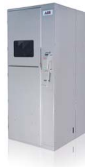
Chain drive handle installed on switchgear
